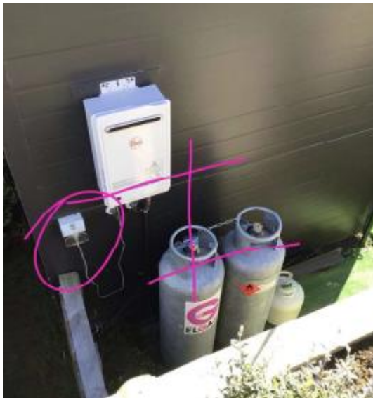
Figure 2 – Sources of Ignition (x2) next to LPG Cylinder Valves 1
