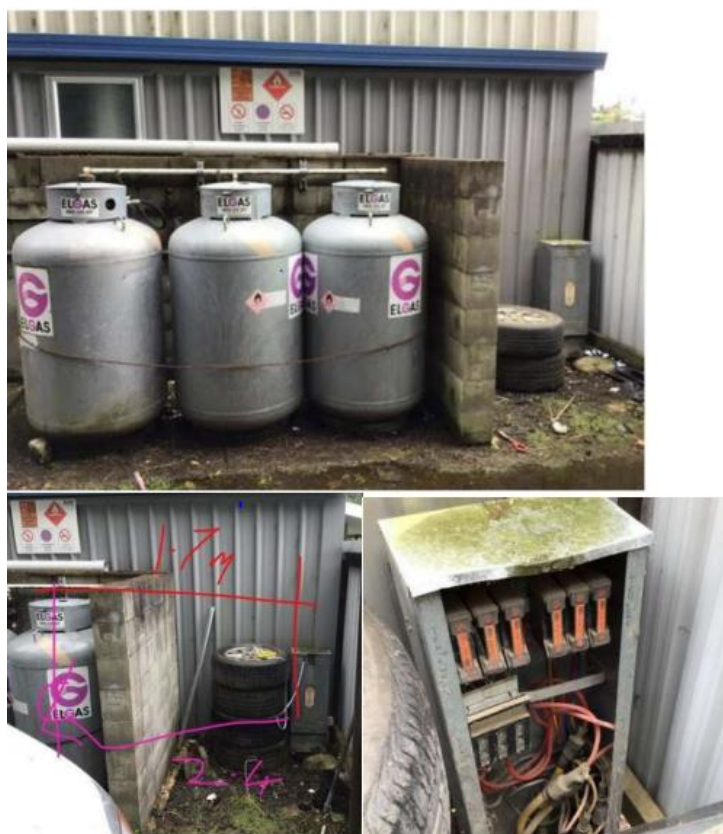
Figure 5 – 66kg LPG location with “high voltage wires” inside the hazardous area
